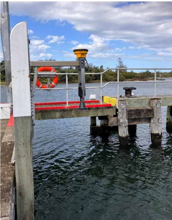
VEGA Probe and Trimble Antenna Installation at Bullock Island.
