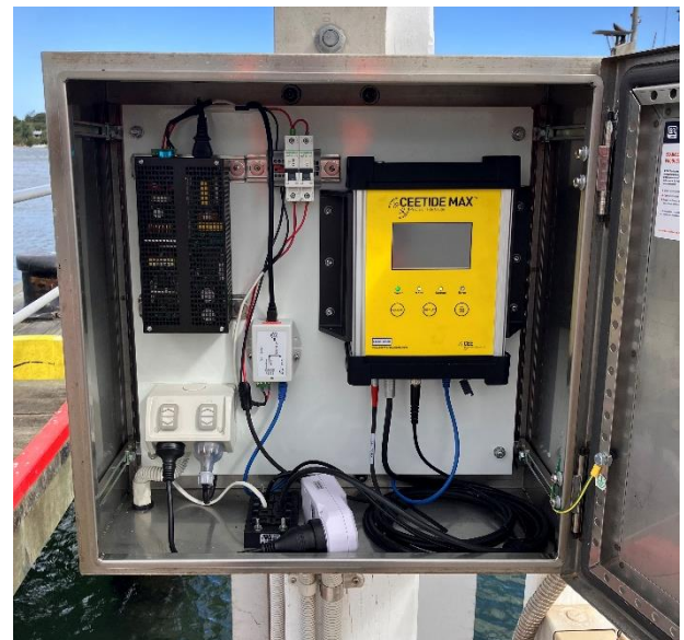
CEETIDE MAX installed at Bullock Island.
